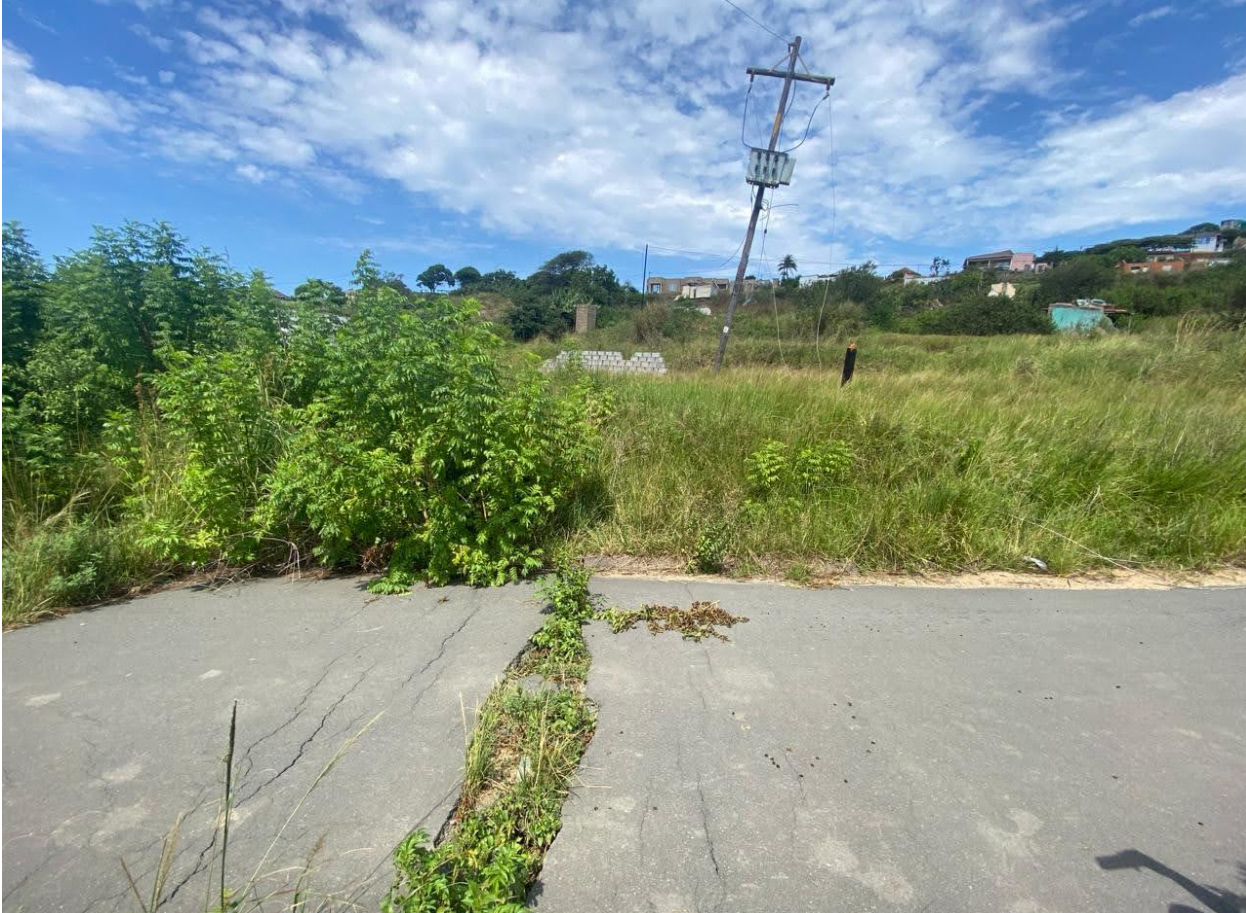
Figure 2: Damaged Electrical Pole and eroded road
