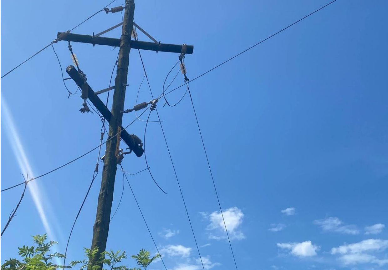
Figure 3: Damaged Power Line
